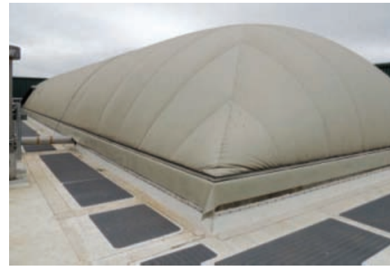
Each bank of eight digesters has its own 425,000 gallon percolate tank in the basement and 670 cubic meter gas storage system on the roof (above).
